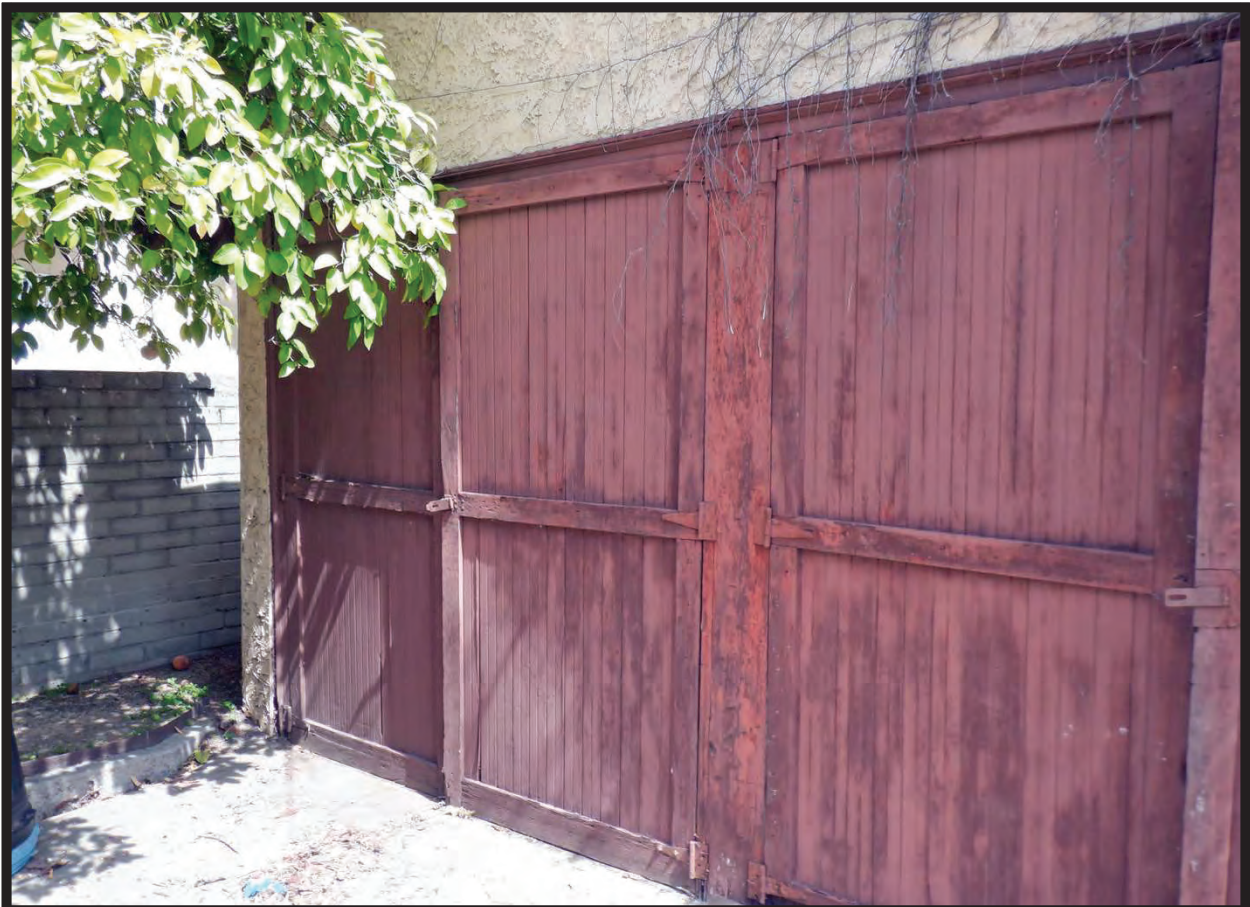
Door Detail, West Elevation of 1926-1927 Garage, 1022 La Cadena Avenue, Arcadia, CA (NE)
