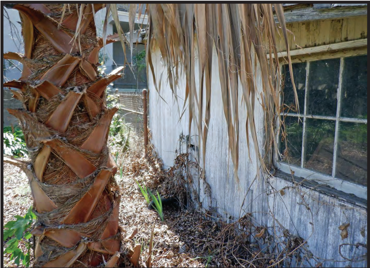
East Elevation of Shed East of 1944 Residence at 1022 La Cadena Avenue, Arcadia, CA (SSW)
