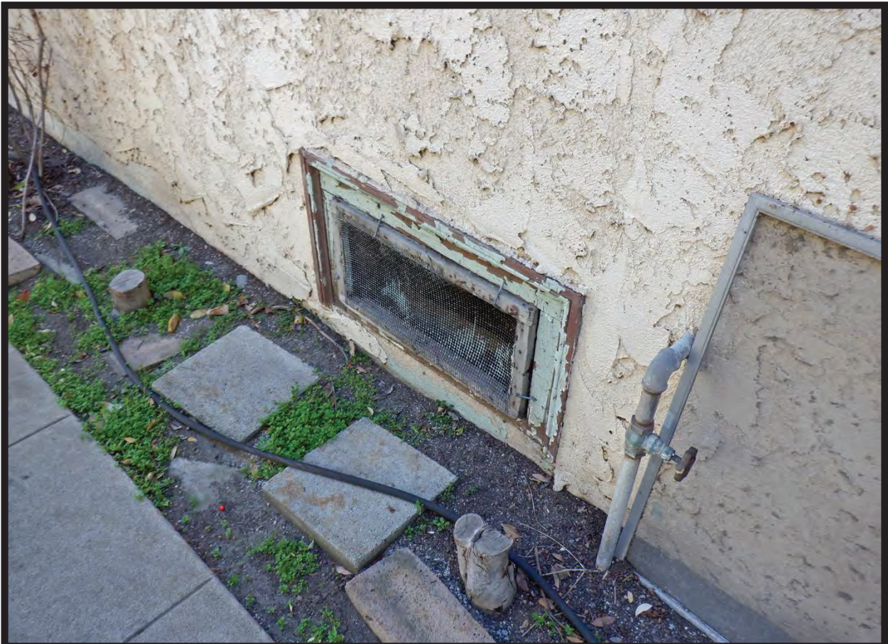
Crawl Space Entrance, North Elevation of Residence at 1022 La Cadena Avenue, Arcadia, CA (SE)
