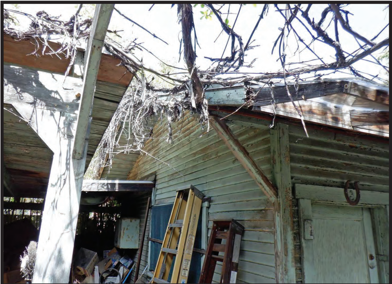
West Elevation of Western Ell of Large Barn/Workshop, 1022 La Cadena Avenue, Arcadia, CA (NNE)
