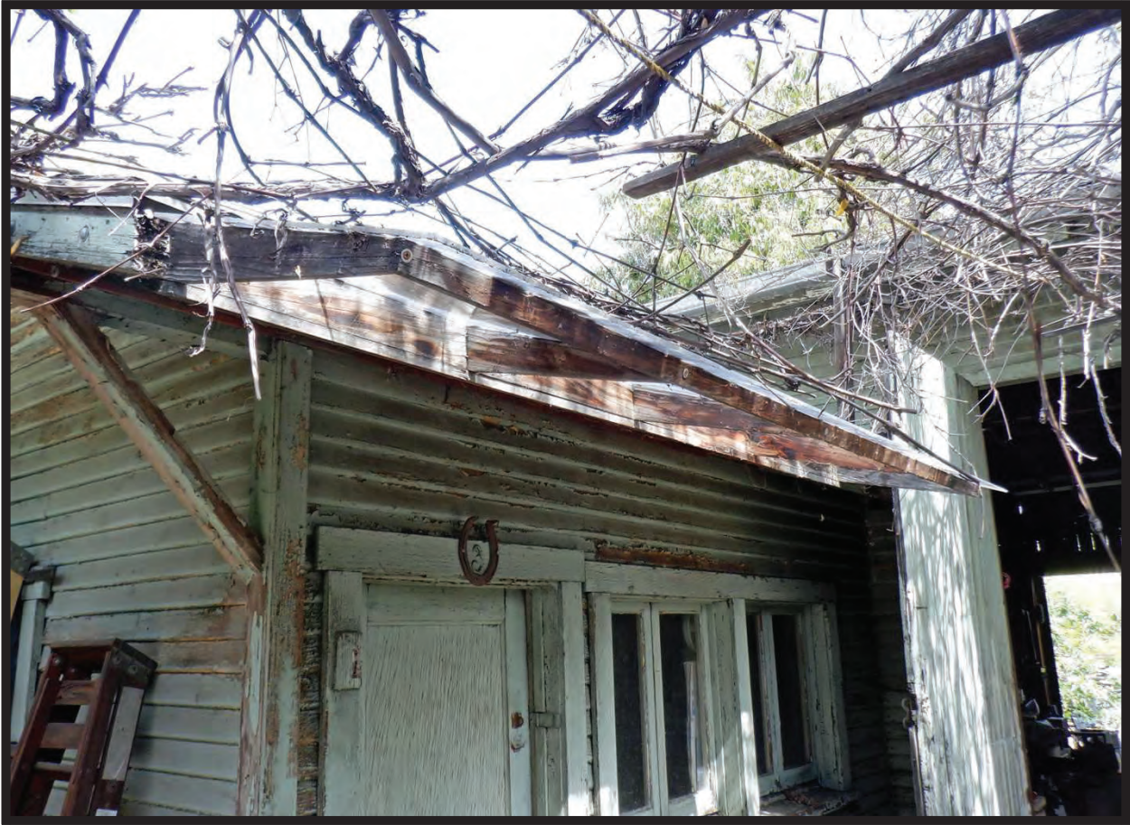
West and South Elevations of Western Ell of Large Barn/Workshop, 1022 La Cadena Avenue, Arcadia, CA (ENE)
