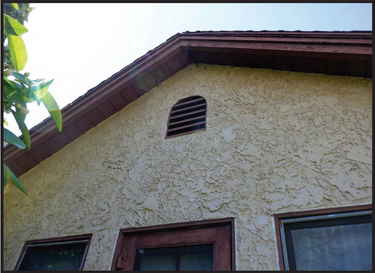
East Elevation of Addition to Residence at 1022 La Cadena Avenue, Arcadia, CA (WSW)
