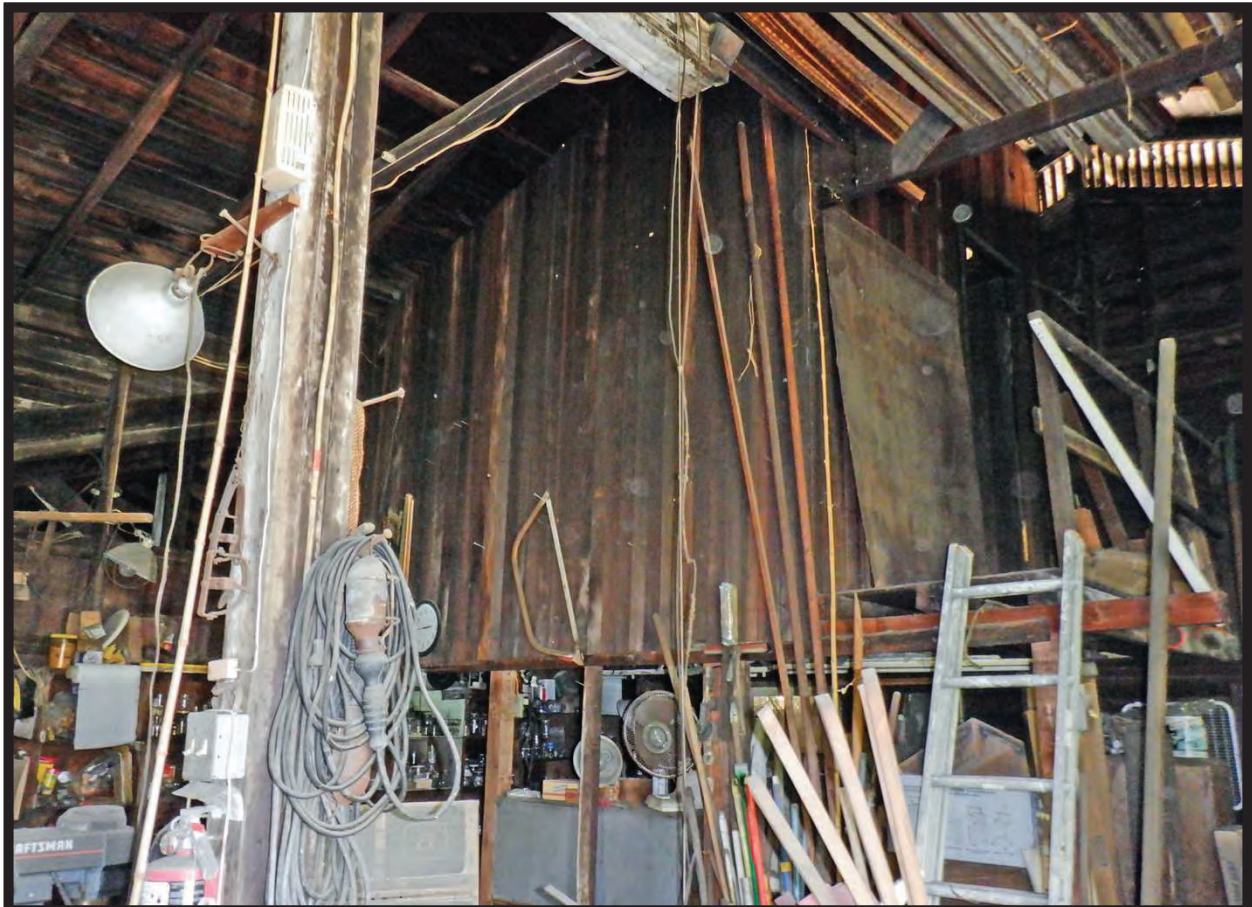
Interior Detail, Large Barn/Workshop with Bay Door, 1022 La Cadena Avenue, Arcadia, CA (NW)
