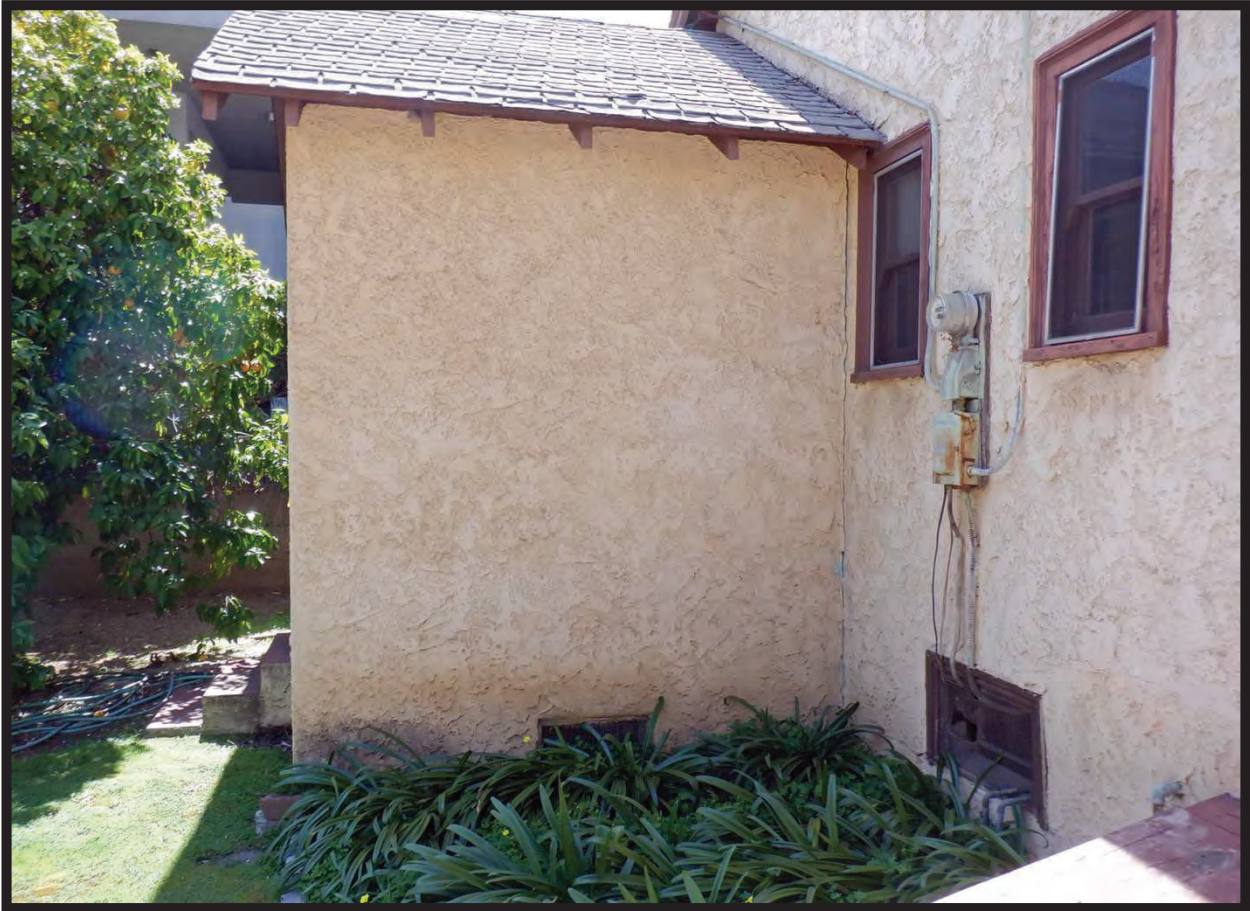
Addition on East Elevation of Residence at 1022 La Cadena Avenue, Arcadia, CA (S)
