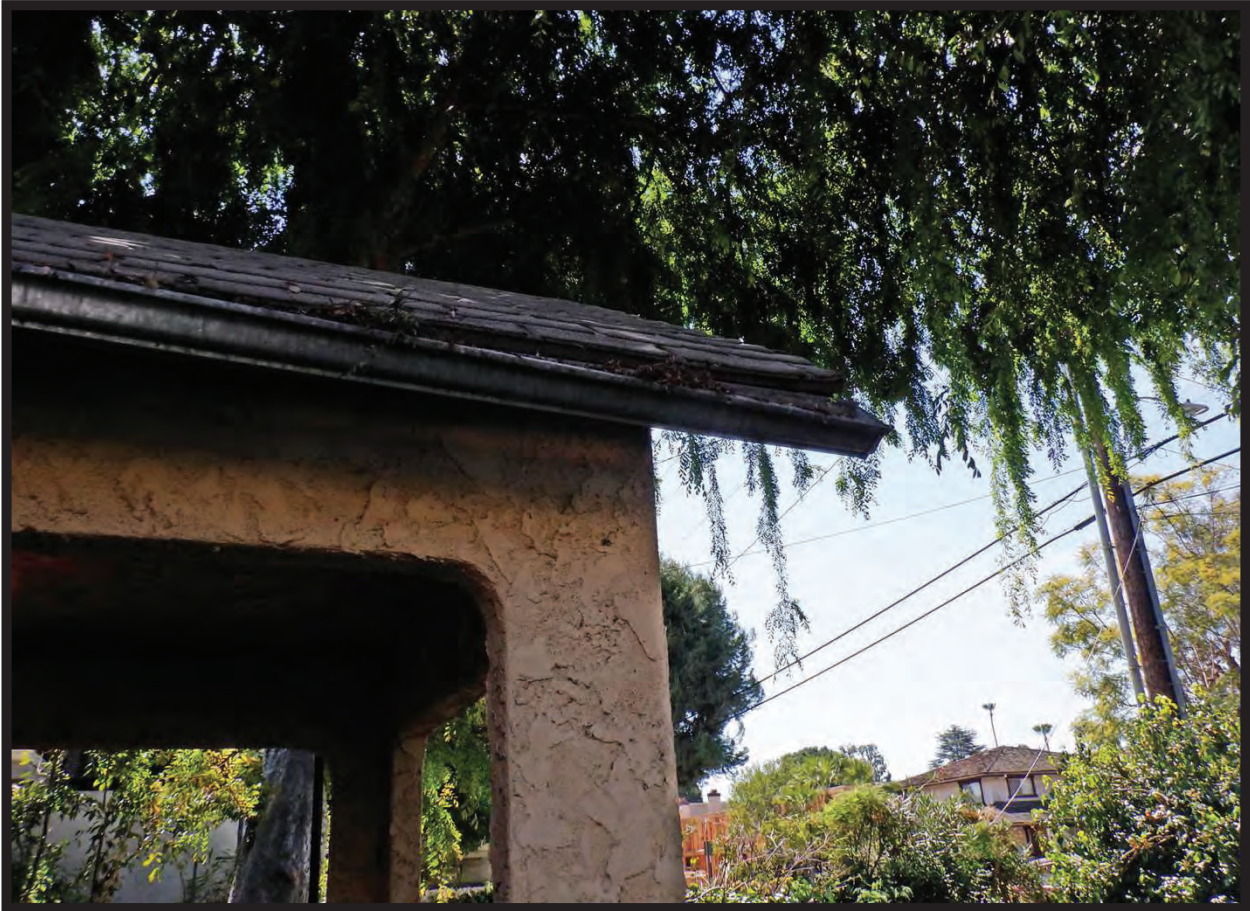
Damaged Eave on West Elevation of Residence at 1022 La Cadena Avenue, Arcadia, CA (SSW)
