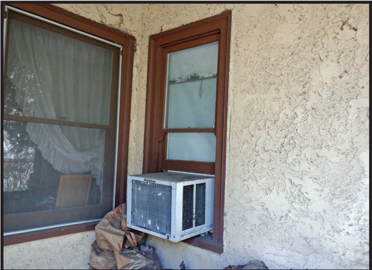
Window Detail, Side Porch, North Elevation of Residence at 1022 La Cadena Avenue, Arcadia, CA (SW)
