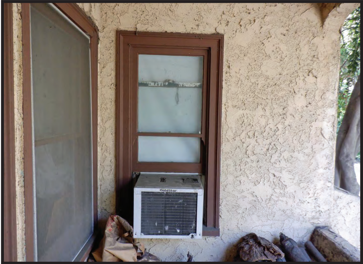
Window Detail, Side Porch, North Elevation of Residence at 1022 La Cadena Avenue, Arcadia, CA (W)
