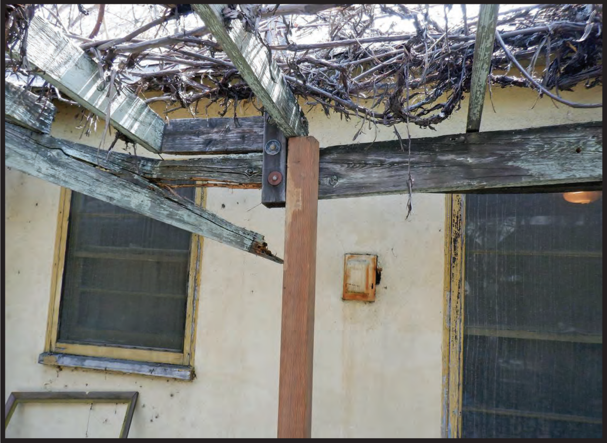
Falling Roof on North Elevation of 1944 Residence, 1022 La Cadena Avenue, Arcadia, CA (S)
