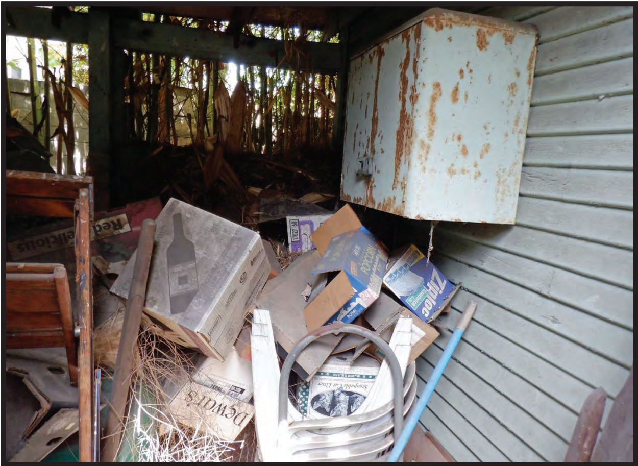
Covered Patio between Office and Garage, 1022 La Cadena Avenue, Arcadia, CA (N)
