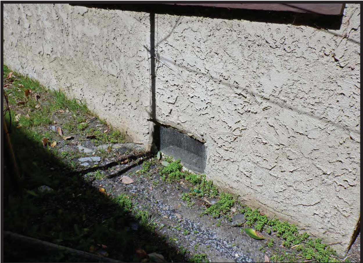
Floor Vent/Crawl Space, South Elevation of Residence at 1022 La Cadena Avenue, Arcadia, CA (NW)
