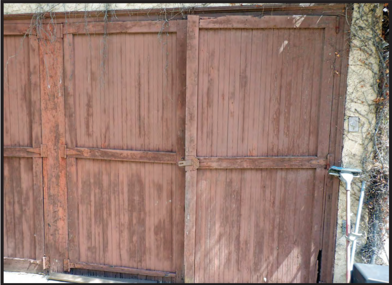
Door Detail, West Elevation of 1926-1927 Garage, 1022 La Cadena Avenue, Arcadia, CA (E)
