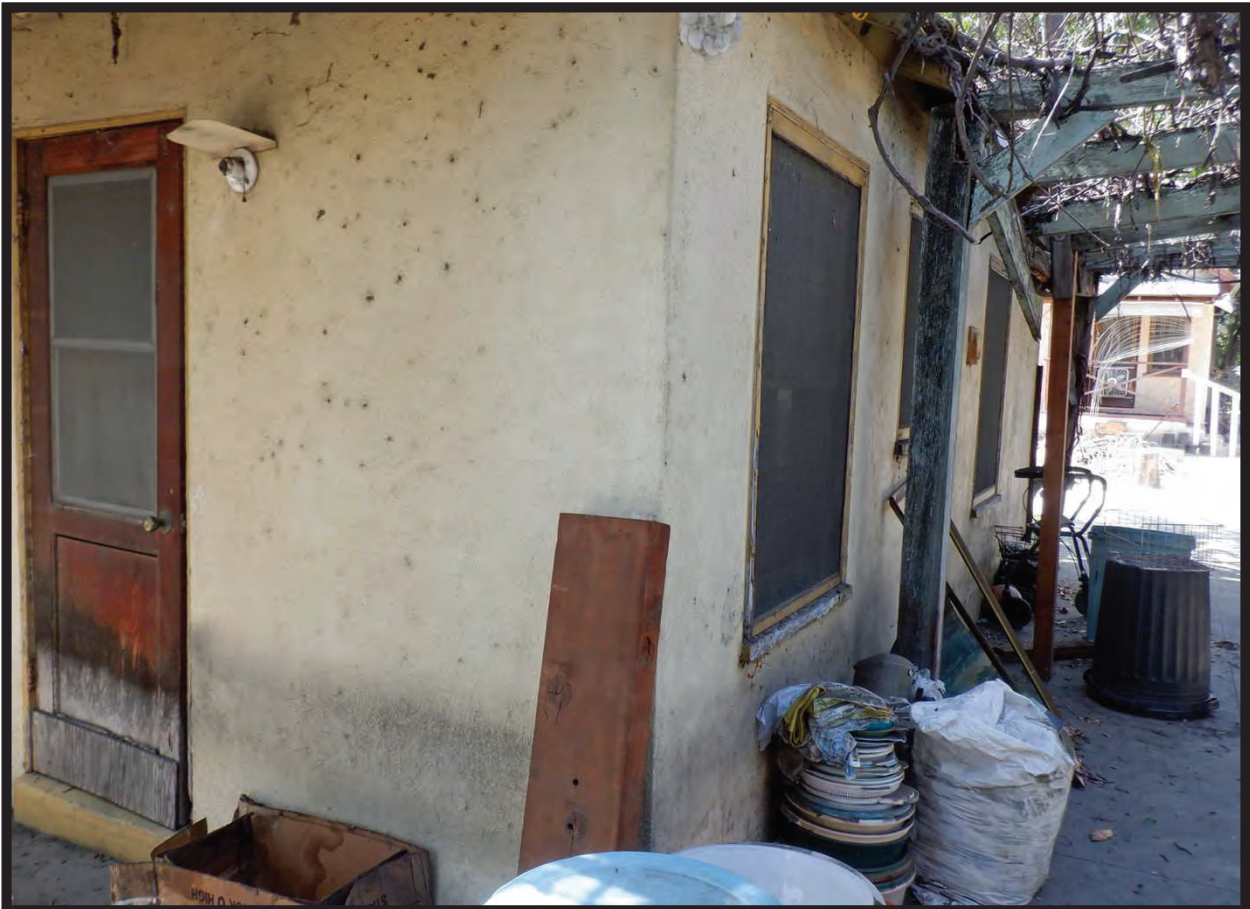
East and North Elevations of 1944 Residence at 1022 La Cadena Avenue, Arcadia, CA (WSW)
