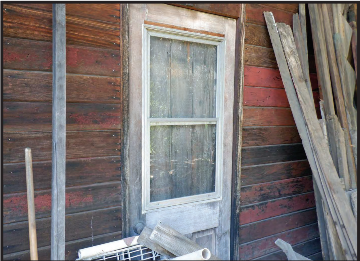
Detail, East Elevation of Large Barn/Workshop with Bay Door, 1022 La Cadena Avenue, Arcadia, CA (NNW)
