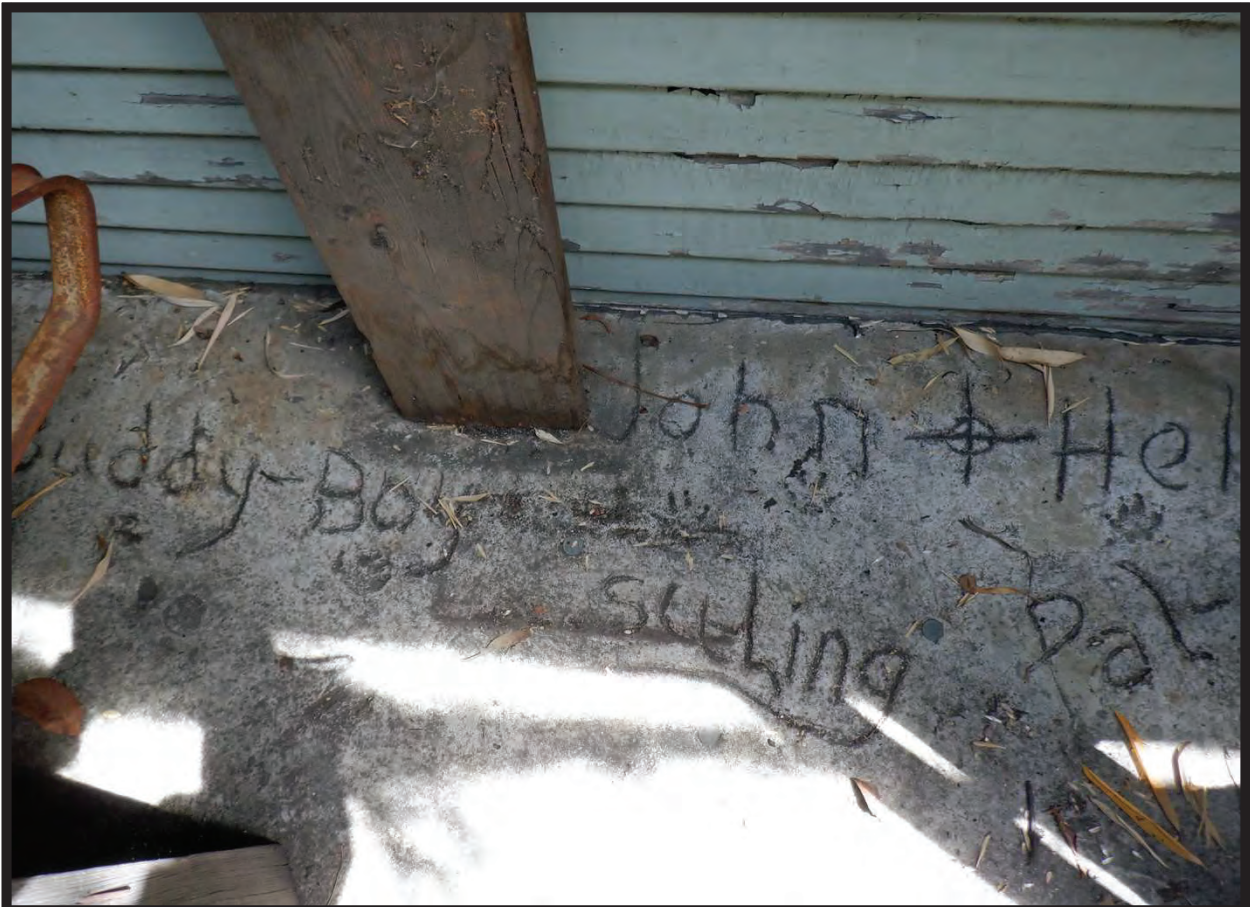
Markings in Concrete to West of Office, 1022 La Cadena Avenue, Arcadia, CA (Detail)
