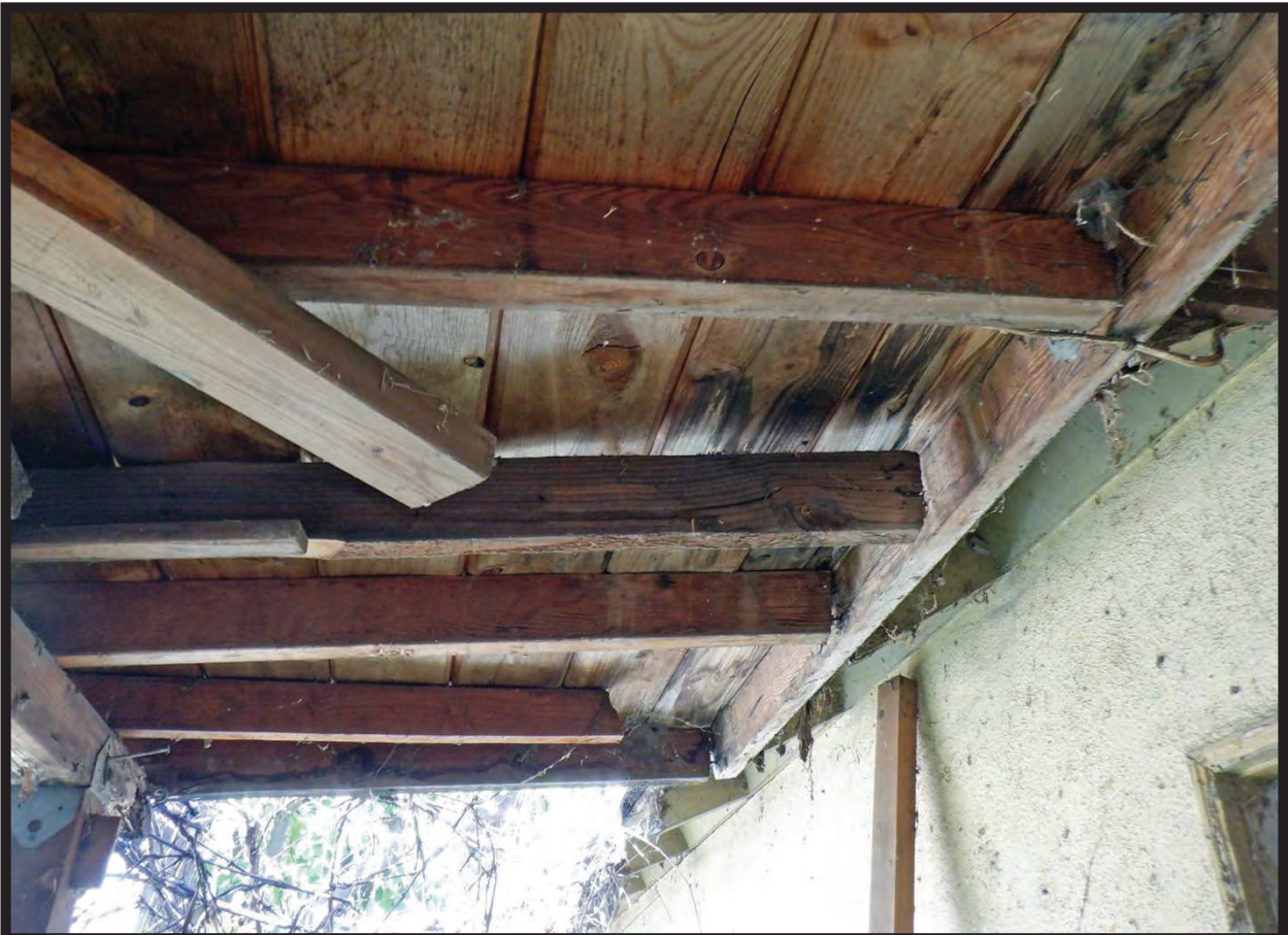
Added Roofing North of 1944 Residence at 1022 La Cadena Avenue, Arcadia, CA (ESE)
