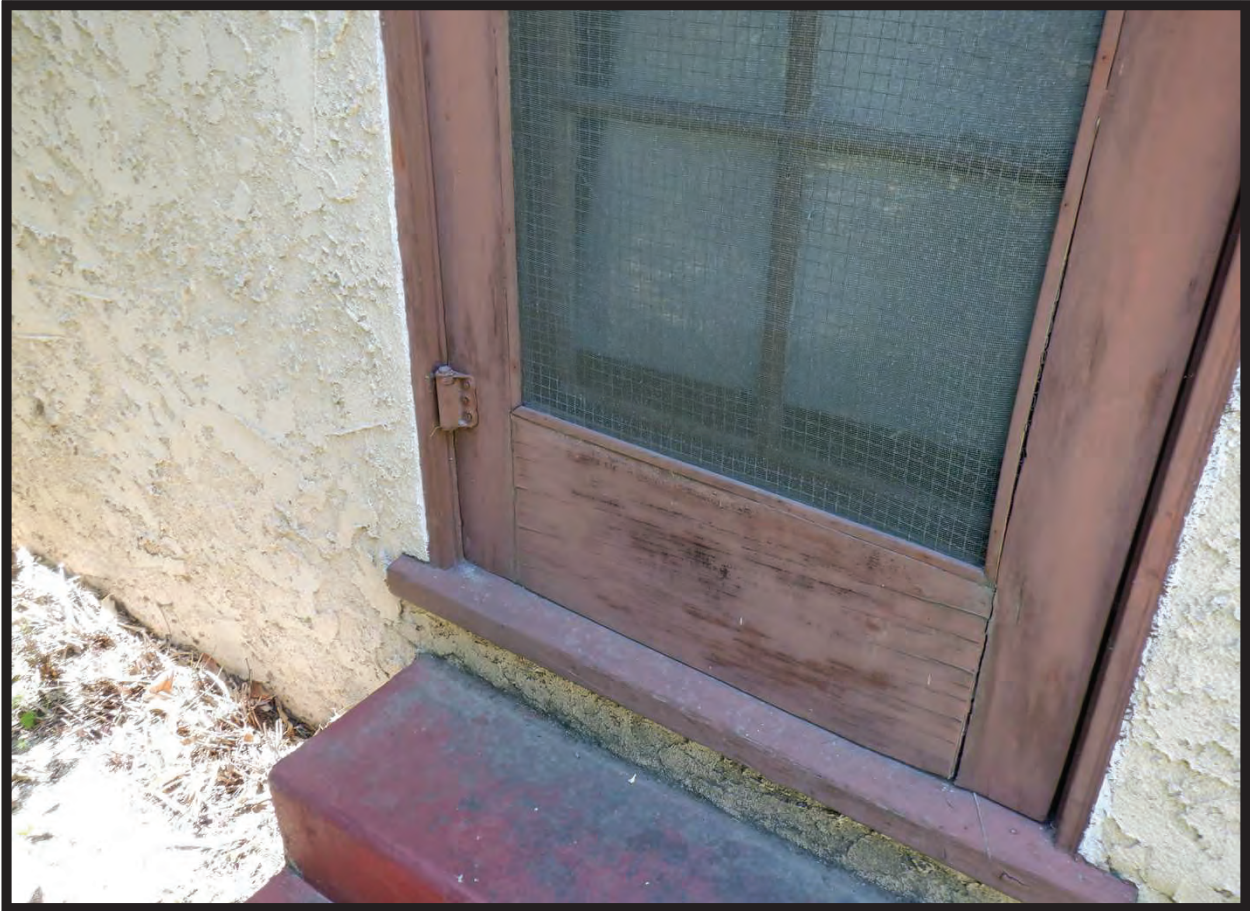
Door and Stoop to Addition on East Elevation of Residence at 1022 La Cadena Avenue, Arcadia, CA (SW)
