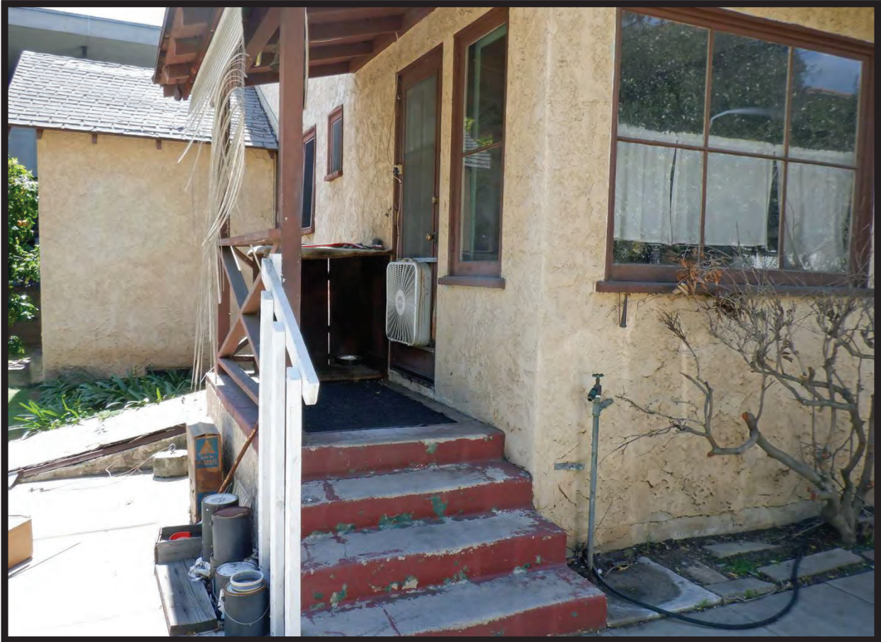
Rear Porch, East Elevation of Residence at 1022 La Cadena Avenue, Arcadia, CA (SSW)
