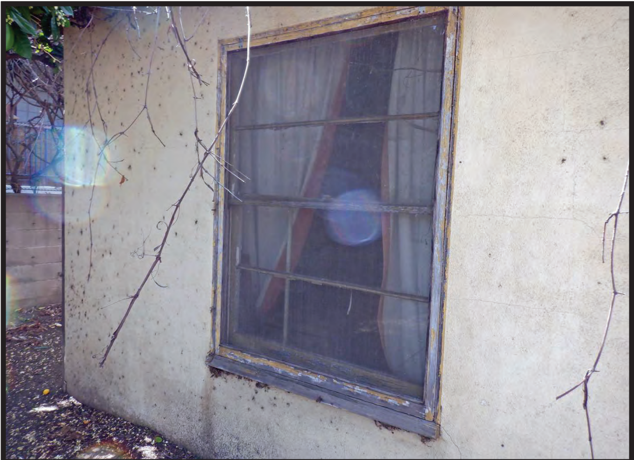
Window Detail, East Elevation of 1944 Residence at 1022 La Cadena Avenue, Arcadia, CA (SW)
