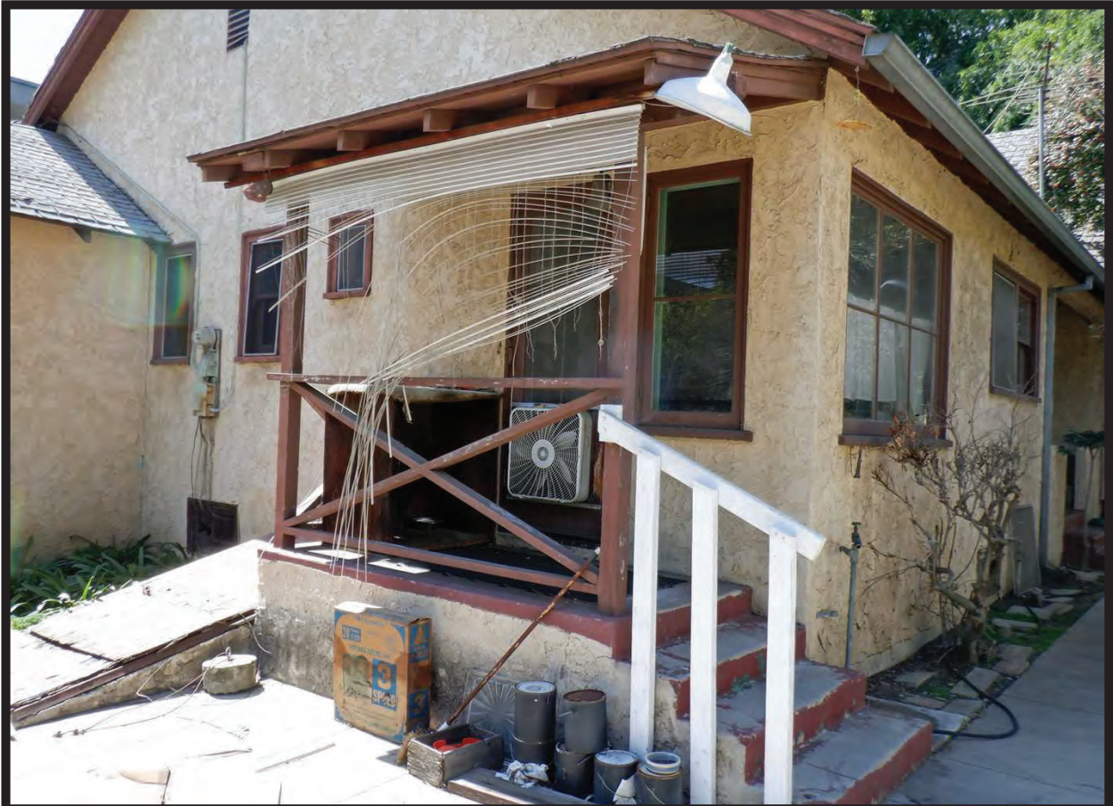
Rear Porch, East Elevation of Residence at 1022 La Cadena Avenue, Arcadia, CA (SW)
