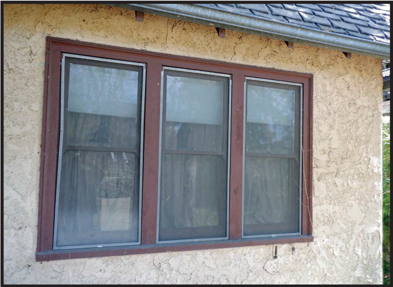
Window Detail, West Elevation of Residence at 1022 La Cadena Avenue, Arcadia, CA (SE)
